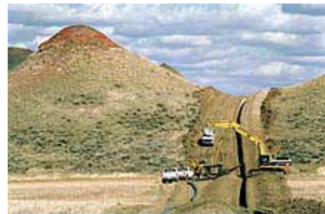
SCARS: Energy workers dig a trench for gas and water pipelines on the Sorenson family homestead in the Powder River Basin (Kevin Moloney photo)
