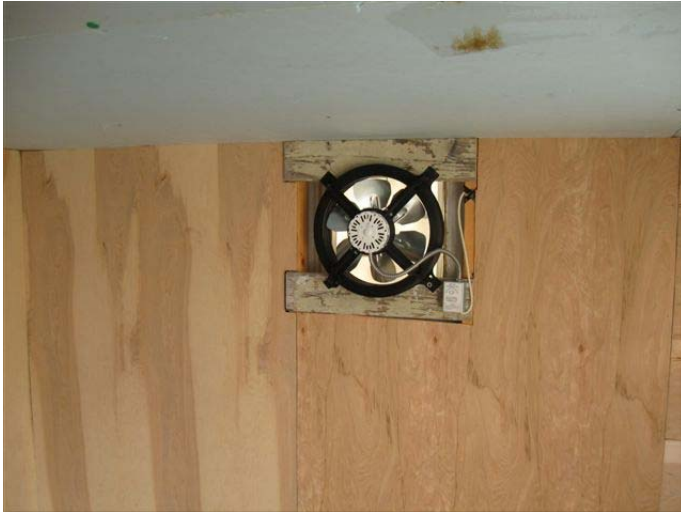
Meg's Place ventilation system
