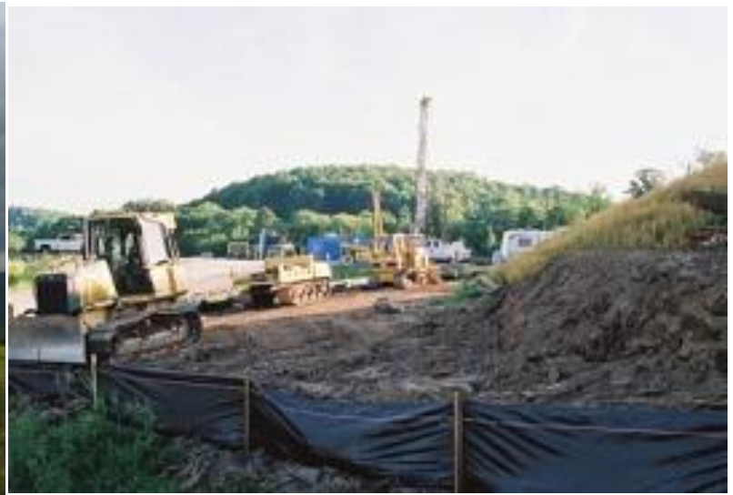
Figure 2: Springville natural gas drilling pipeline in Pennsylvania Flickr user “arimoore” taken by Helen Slottje for Shaleshock Used under Creative Commons Attribution-NonCommercial-ShareAlike 2.0 license.
